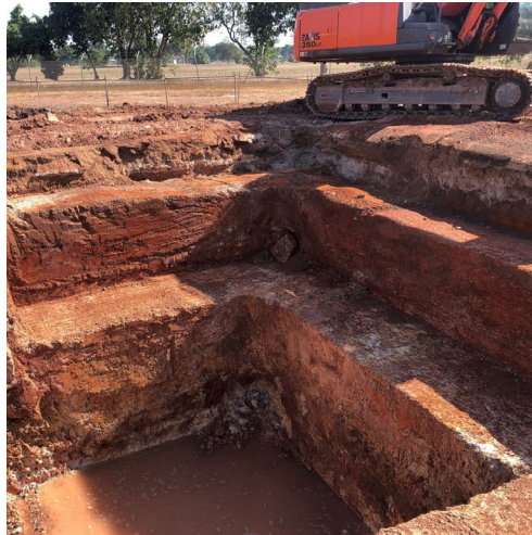
Sewer pump chamber
