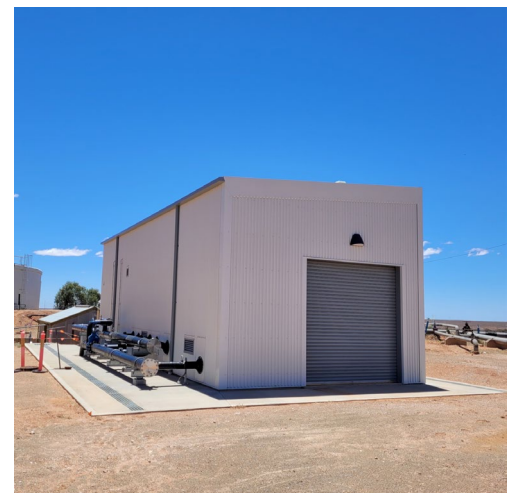
New pump house
