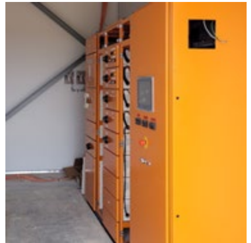
New main switchboard
