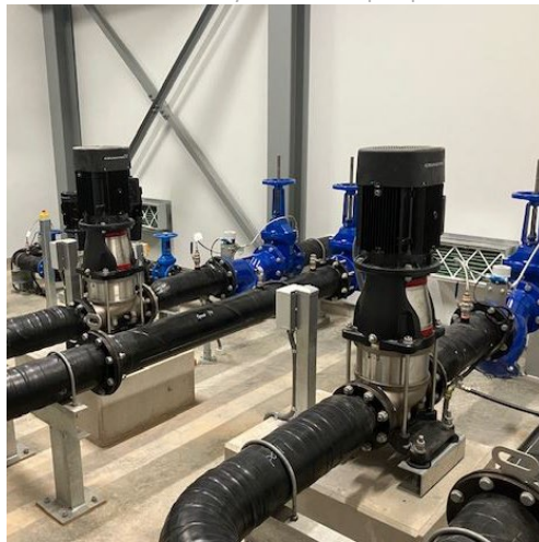
Pump system installed
